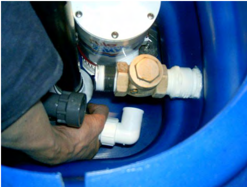
PLUMBING ASSEMBLY REMOVED
