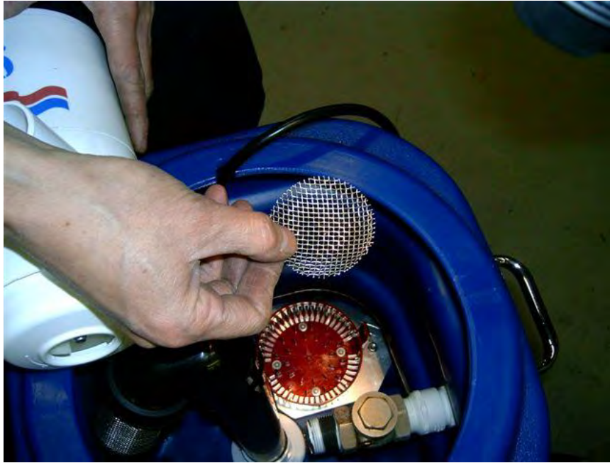
S.S. SCREEN LIFTS OUT OF STRAINER CAGE TO BE CLEANED
